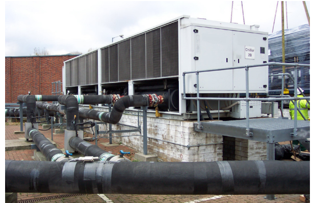
Before: The existing chiller before the arrival of the Turbomisers
