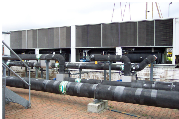
Before: The old chillers had become inefficient and subject to breakdowns
