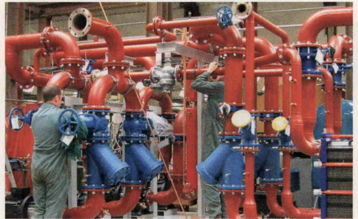
The move to offsite fabrication has led to successful business for Ormandy over the last 10 years.
