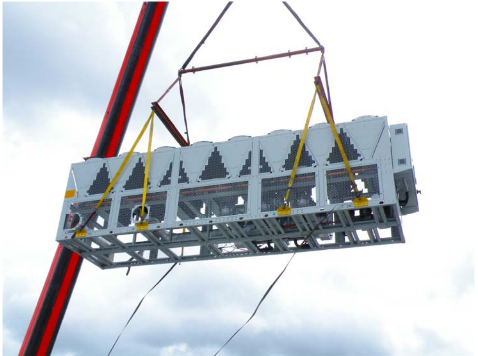
One of the replacement Turbomiser chillers is lifted into position on the rooftop
